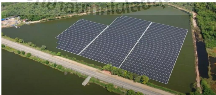
Figure 3.3 Floating PV power plant at SUT
