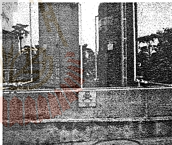
50 % NAOH TANK & 32% HCL TANK
