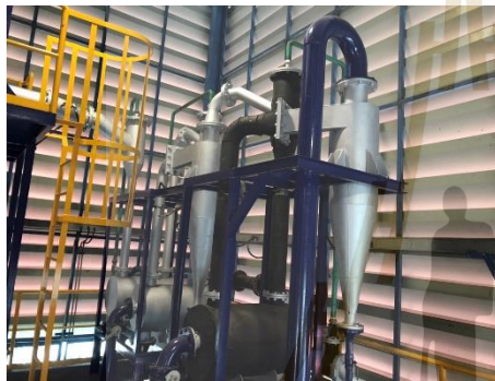
ค. Water scrubber and Chiller scrubber Unit
