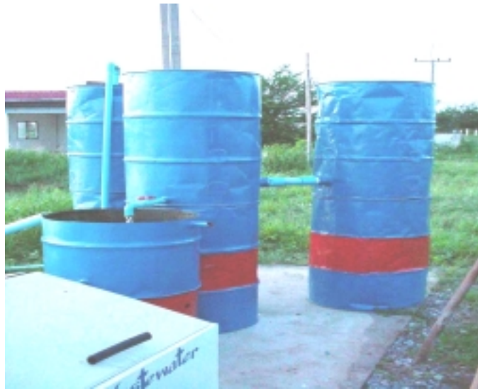
Figure 3-5. Head tank unit.
