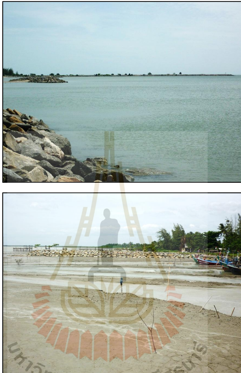
Figure A-14 The jetties, breakwaters, and groins in Ban Tha Sung Bon and Hat Dan Phasi,(taken on 18/07/2012).
