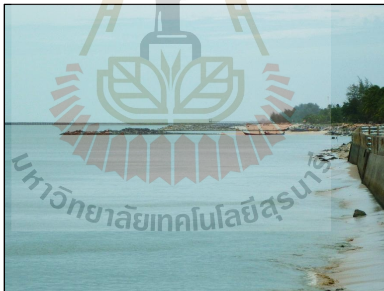
Figure A-30 Breakwaters in southern part of Ban Na San (taken on 19/07/2012).
