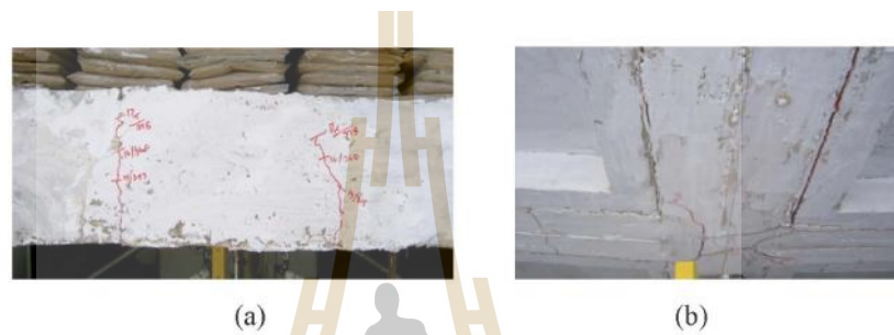
Figure 9 Concrete cracking at the joint interfaces
