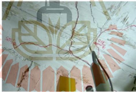
Figure 10 Concrete cracking at mid-span
