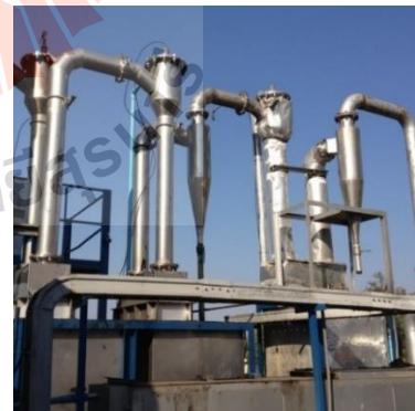
ฉ. Water Scrubber and Chiller Scrubber
