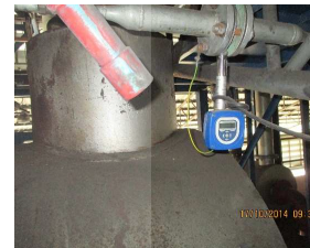
ฉ. Steam Flow Meter
