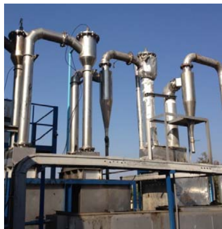
ข. Water scrubber and chiller scrubber
