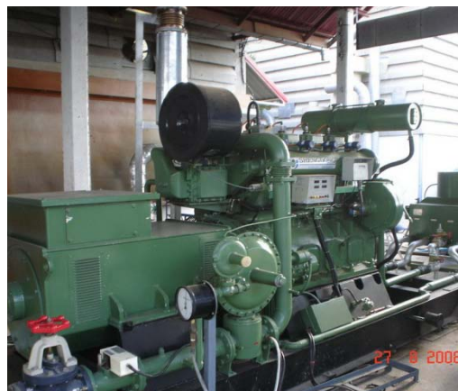
ฎ. Gas-engine Generator Set
