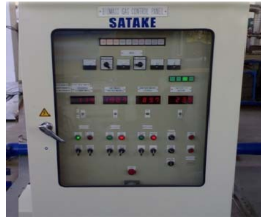
ญ. Biomass Gas Control
