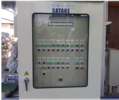
ณ. Biomass Power Plant Control
