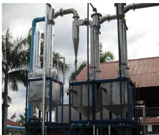
ค. Water Scrubber and Chiller Scrubber
