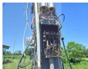
Fig. 1. Lighting control relay and safety switch.
