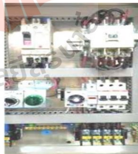
Fig. 2. Lighting control panel with magnetic contactor.
