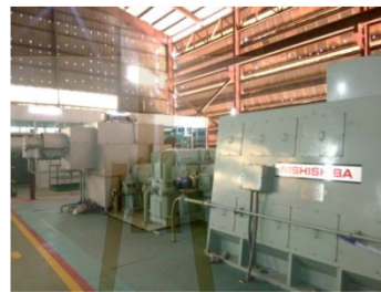
Fig. 5. Steam turbine-generator brand SHINKO with 9 MW capacities.
