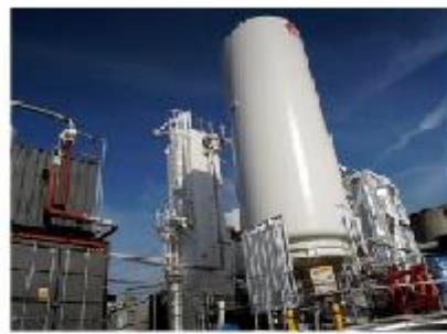
Liquid Air Energy Storage System
