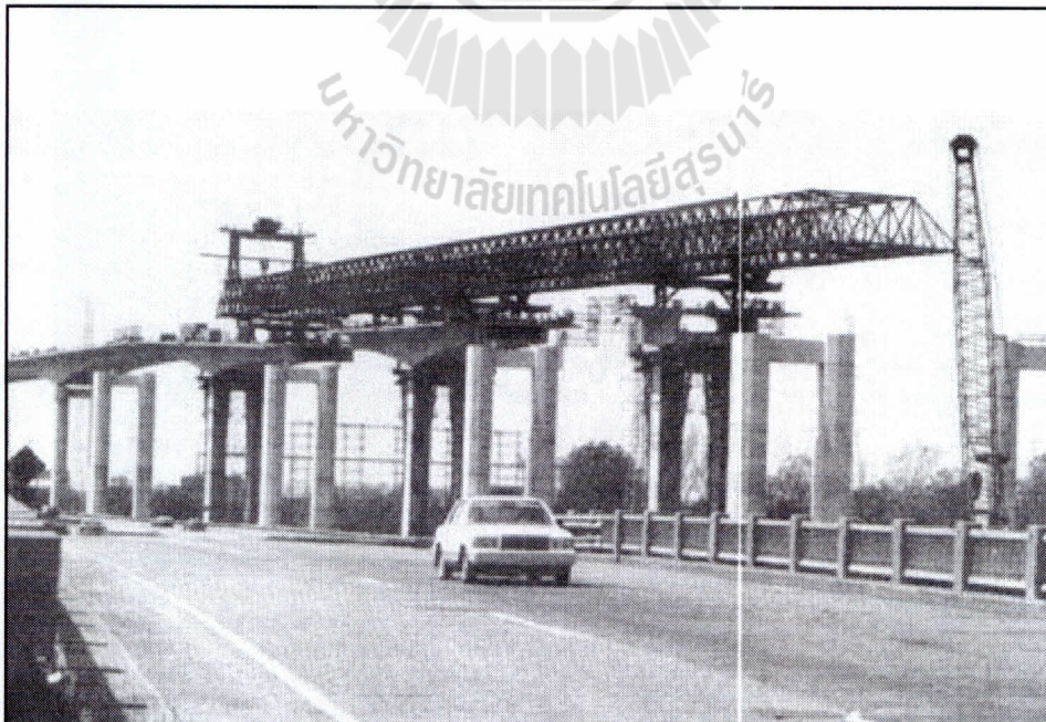
A construction accident at the bridge caused a 300-foot section of the bridge deck to sag five feet at one end and rise three-and-a-half feet at the other.
