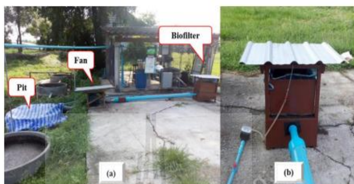
Fig. 1. The system which include a covered pit, a fan, a piping system, and a biofilter unit (a), and the close-up of the inlet side of tray biofilter, with the automatic water spraying system on the left (b).
