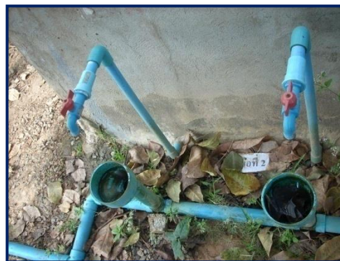
Figure 3.4 Water outlet of subsurface flow constructed wetlands.
