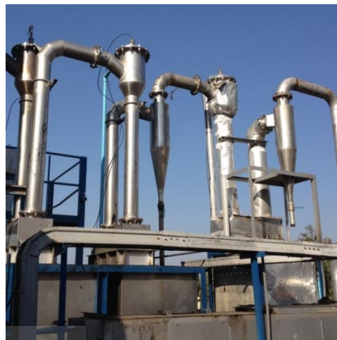
ฉ. Water scrubber and chiller scrubber
