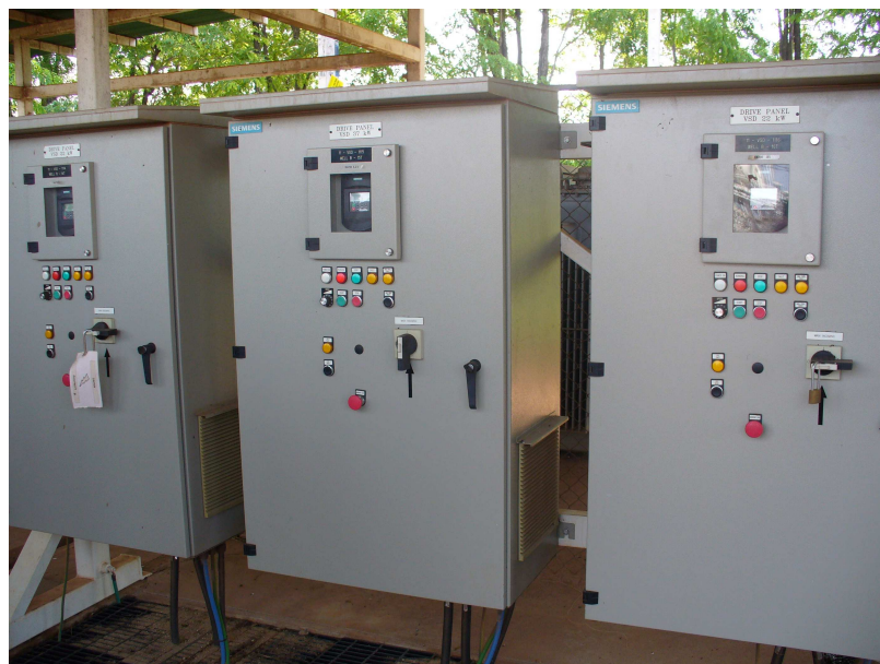
Figure 2.16 Whetherford's controller of electrical submersible pump in Sirikit oil fields.
