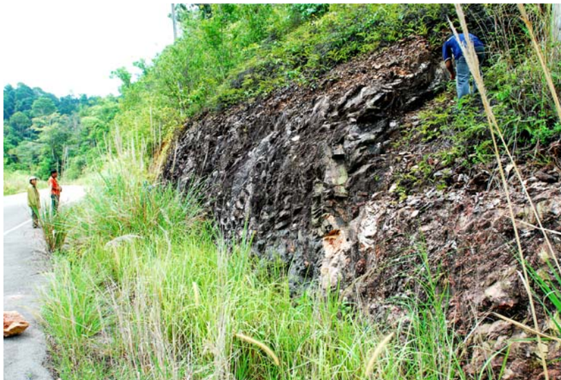
Figure 3.5 Micaceous siltstone collected from the embankment of Khao Chuk reservoir in Rayong province.
