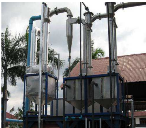
ค. Water Scrubber and Chiller Scrubber Unit
