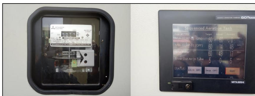
Figure B.9 Wastewater treatment kWh meter and control panel. The control panel shows operation time of CAT, SAT, and transferring pumps.
