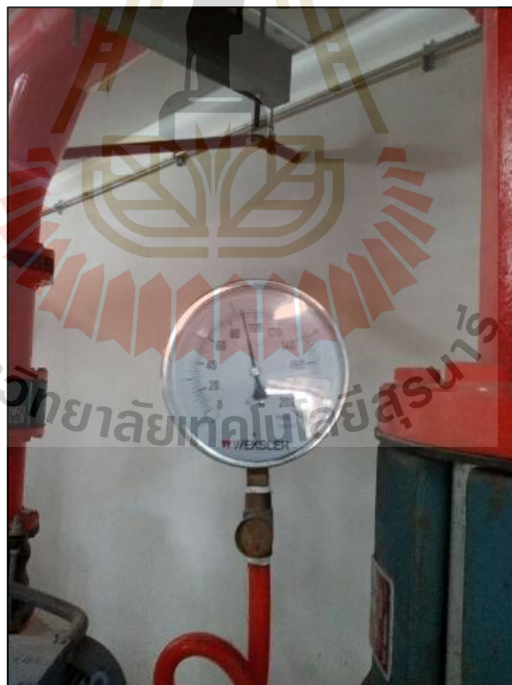
Figure B.8 CDP pump gauges.
