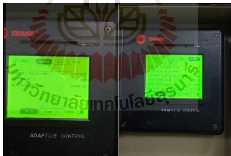
Figure B.6 Control of the chiller showing voltage and current at the chiller, and condenser inlet and outlet water temperature.
