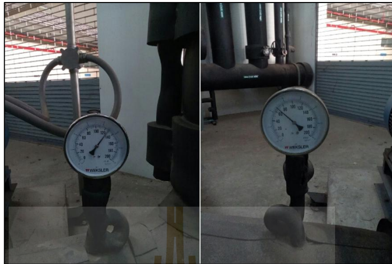
Figure B.7 CHP outlet and inlet pump gauges.
