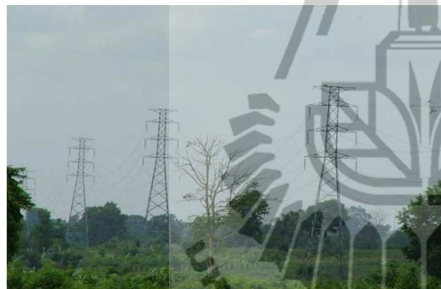
Fig. 2 Electric power transmission line in Nakhon Ratchasima
