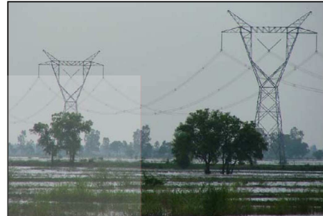
Fig. 3 Electric power transmission line in Nakhon Swan
